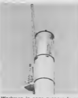
Workers in cage prepare to remove corroded stack section. Trahadornan den baki ta prepara pa desmantela seccion trustiá di e schoorsteen.
